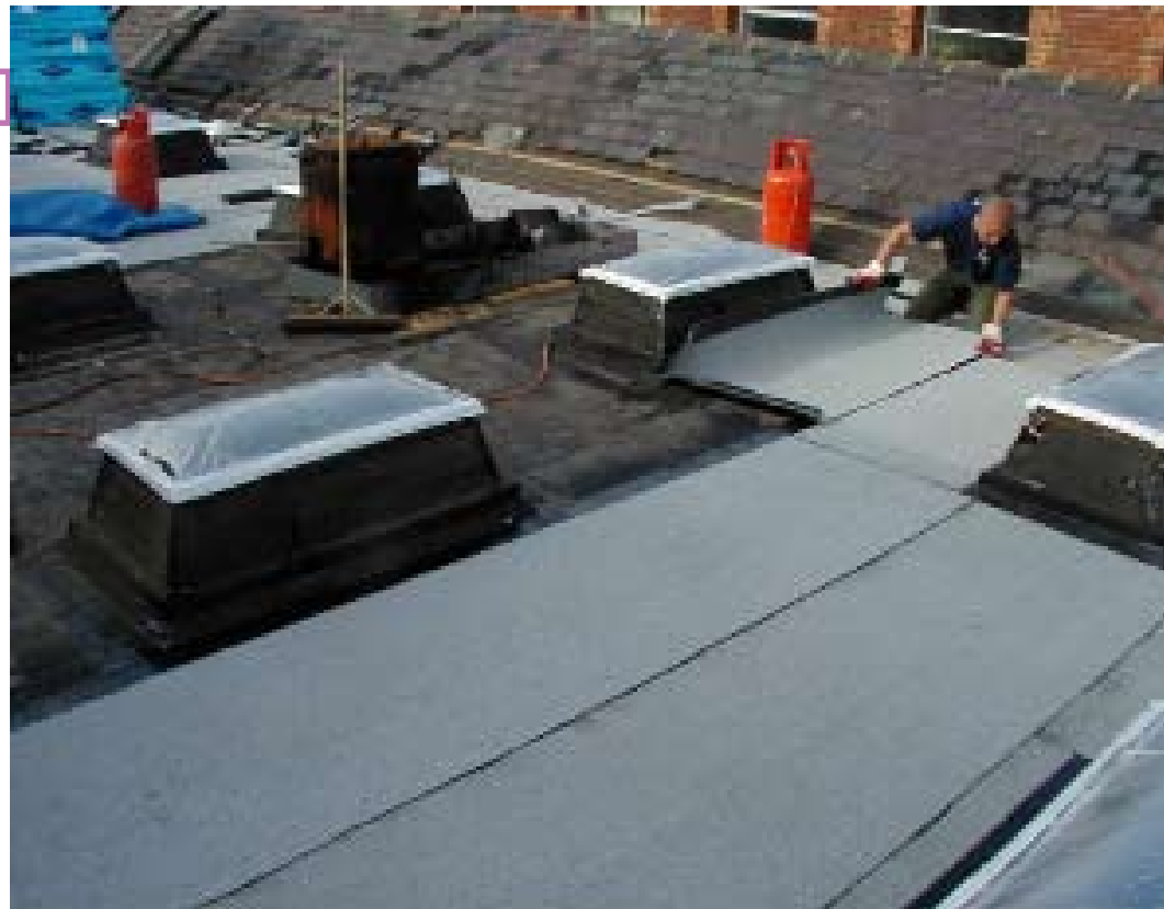
3. STRENGTHENING TO SPREAD LOAD EVENLY & COVER WITH SPECIAL DRAINAGE AND ROOT REPELLENT
